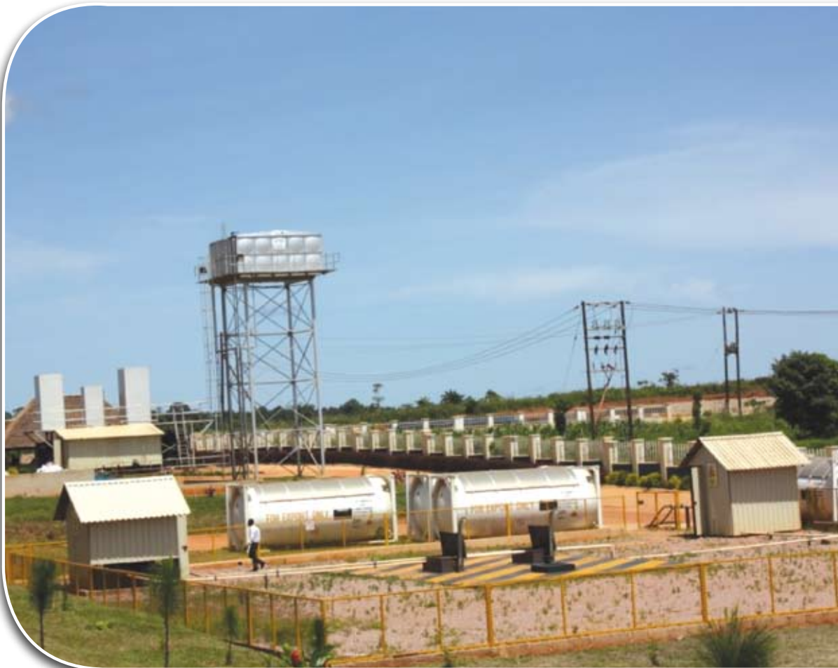
The Thermal Power plant at Namanve Industrial Park
